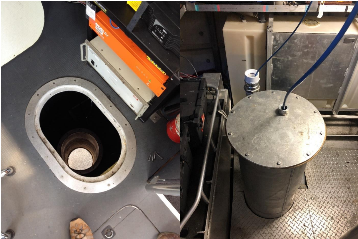
Figure 15. Access to the MBES transducer well as seen from the access hatch in the main cabin deck floor (left) photographed in 2014. Installed MBES and SVS (right) with transducer cover secured photographed during the 2022 MAC. During transit the MBES remains deployed, however, the SVS device is recovered.
