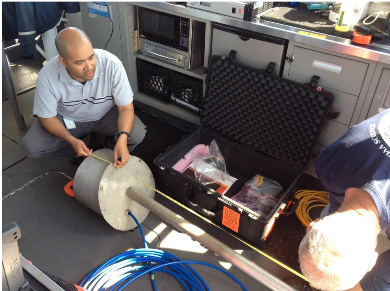
Figure 16. Reference measured between the MBES transducer phase center and the top of the mounting flange which secures the unit inside the transducer well. Image from 2014 sonar installation.
